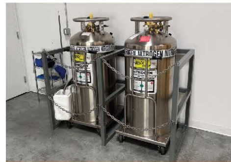
Gas Cylinder Storage
